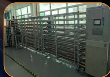
Automatic conveying and drying equipment
